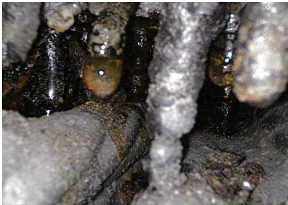
This image shows a duct with exposed tendons in the duct interior. Note the mineral and water deposits. (Photo courtesy of VSL)
