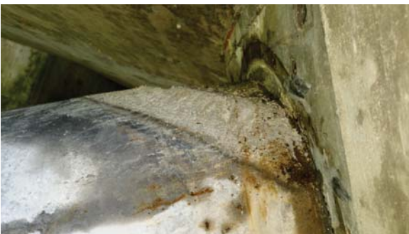
Soft grout can be seen at the anchor of the steel tendon pictured here. (Photo courtesy of VSL)
