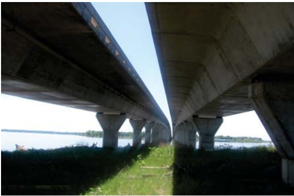
US 59 post-tensioned bridges over Grand Lake in Delaware County, Oklahoma. (Photo courtesy of SCS)
