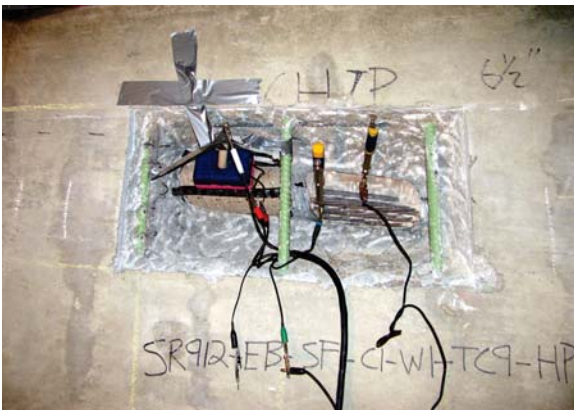
A corrosion rate setup for an interior steel tendon. (Photo courtesy of SCS)
