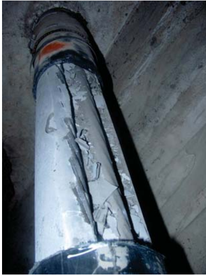
This exterior tendon has a large void. Note that the steel tendon is exposed. (Photo courtesy of SCS)
