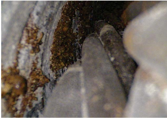
This tendon duct has no grout. Note that there is rust on the duct interior and the steel tendon strands. (Photo courtesy of VSL)
