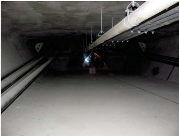
A typical view of external tendons in a post-tensioned structure. (Photo courtesy of SCS)
