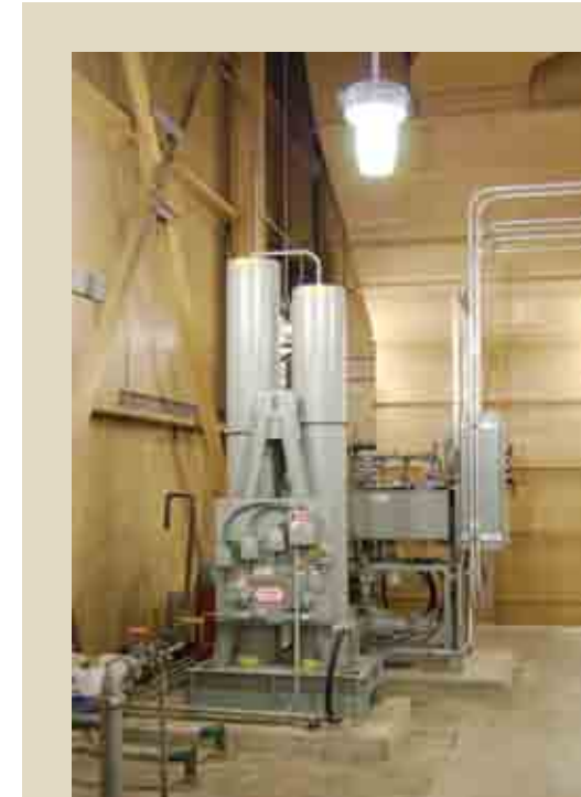
Pictured Left: A new hydraulic power package and accumulator allow the 96-inch influent gate to open under 68 feet of differential pressure. This includes a new hydraulic cylinder that operates under 3000 psi hydraulic pressure to open the gate in 3 minutes and close it in 60 seconds in case of an emergency condition.
