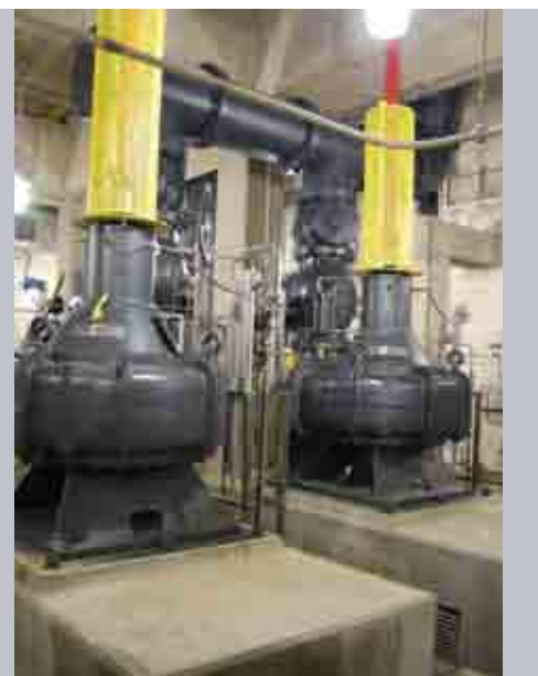
Pictured Right: Low-flow pumps will handle dry weather flows.
