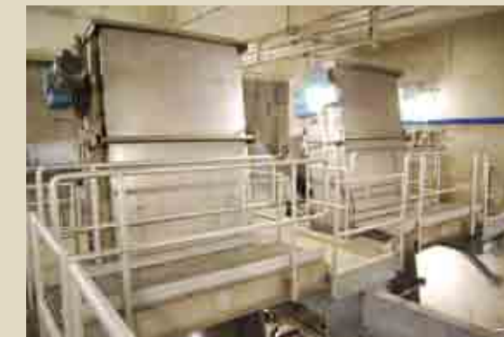
Pictured Left: The headworks bar screen and new service platform enhance operator safety.
