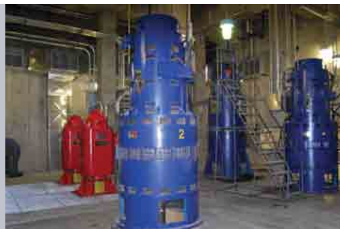
Pictured Above: Two new 250 horsepower (HP), low-flow pump motors (red) work with existing 800 HP motors (blue). All pumps are equipped with variable speed drives to match incoming flows, conserve energy and extend pump life.
