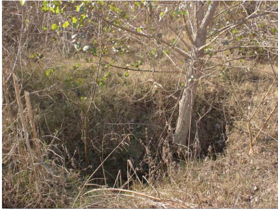
Figure 11.0 – Picture of sinkhole.
