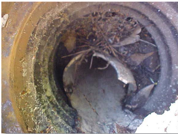
Figure 12.0 – Picture of pipe collapse/failure with root intrusion.
