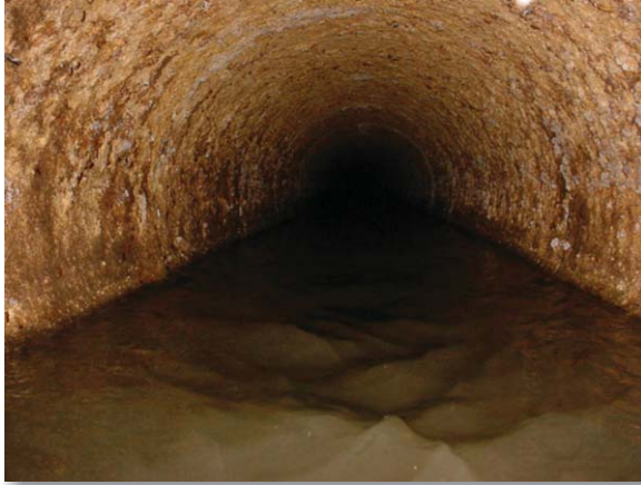
Figure 14.0 – Interior picture of wastewater pipe deteriorated by H2S
