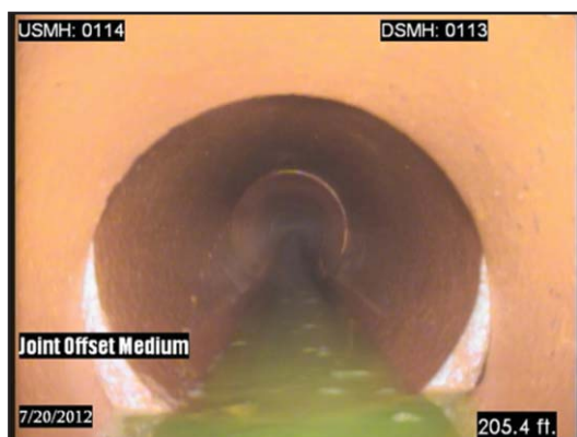
Figure 2.0 – Internal Pipe Image of Dye Test infiltrating through an open pipe joint.
