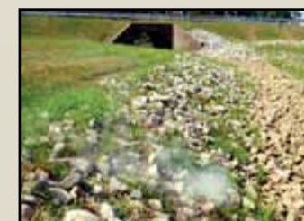
Smoke testing is a tool that can be used for determining public and private I/I pathways.
