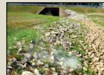
Smoke testing is a tool that can be used for determining public and private I/I pathways.
