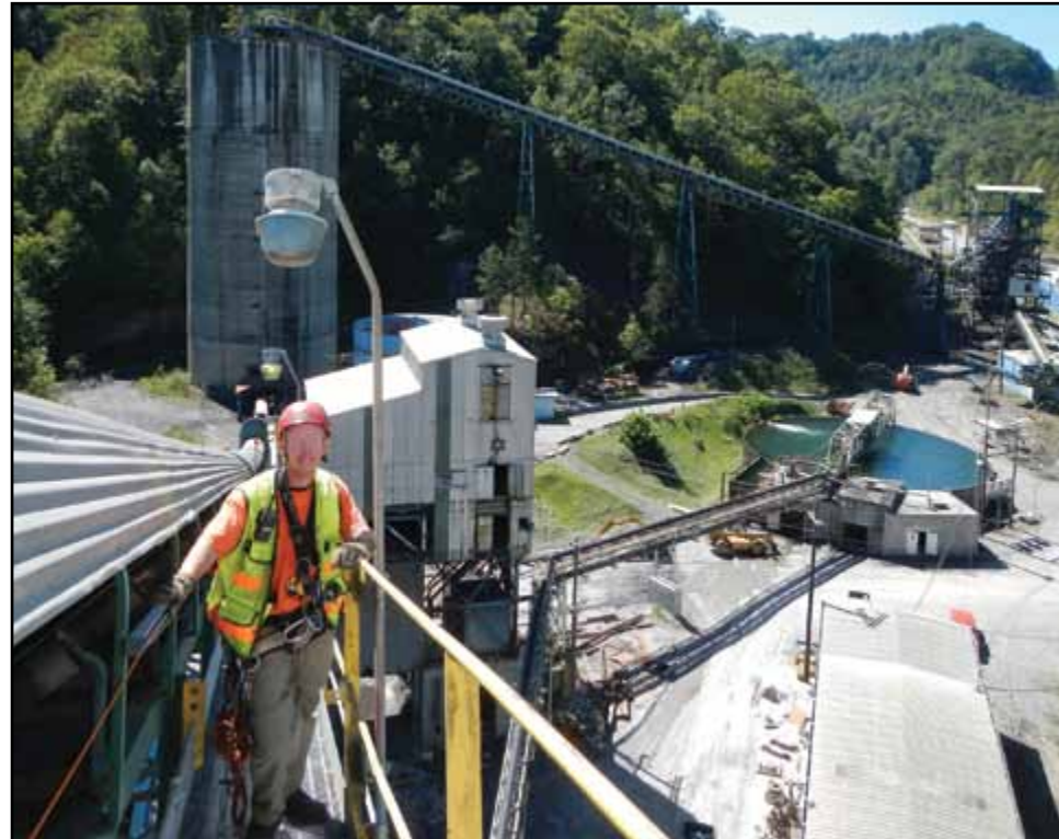
B&N engineers inspected the aboveground mining facilities and identified solutions to improve structural integrity.
